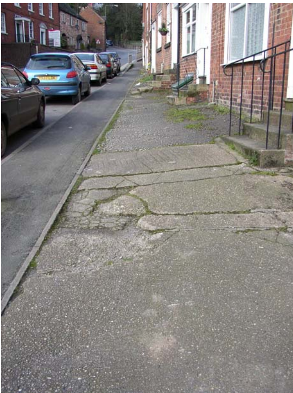
6. Unattractive broken concrete apron to properties at the junction with King Street (north).
